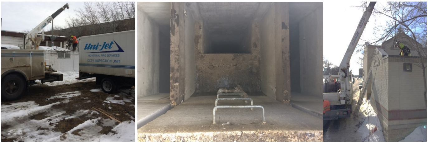
Figure 17: Working at Height and Access Issues
